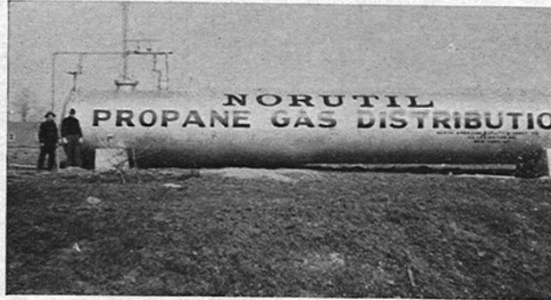
Central Storage Tank for Gas System
